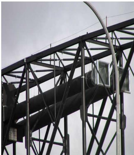
VECTOR ARENA ROOF STRUCTURE AND AIR CONDITIONING DUCTING
